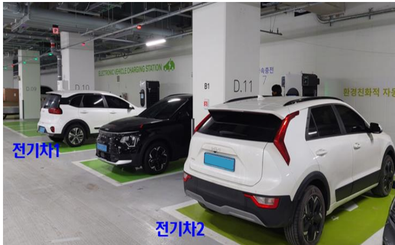
지하 1층 전기차 충전소 (Electronic Vehicle Charging Station)
